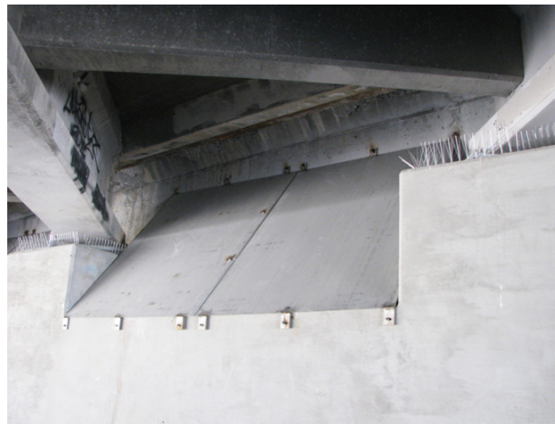
Figure 23. North Diversion Channel, Indian School Bridge Avian Control Project - Bird Spikes and Spiders
