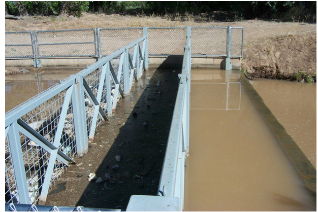
Figure 13. La Orilla Outlet Debris Baffle
