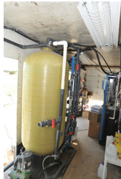
Figure 6. Softening Tank (Ion Exchange)
