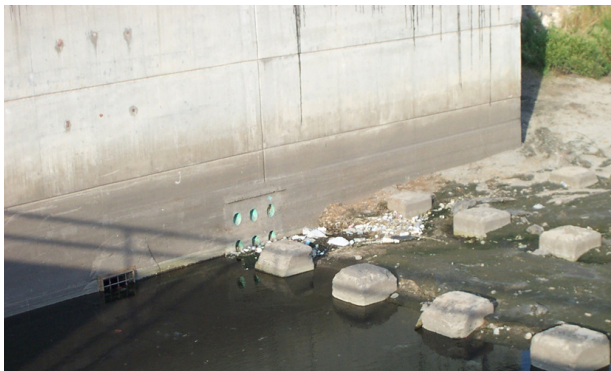
Figure 25. North Diversion Channel "Bathtub" Drains
