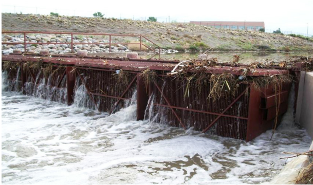
Figure 15. Bear Canyon Arroyo Debris Screen
