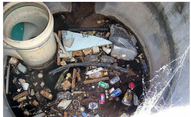
Figure 14. By-Pass Manhole Debris Containment after One Year of Operation and Before Maintenance
